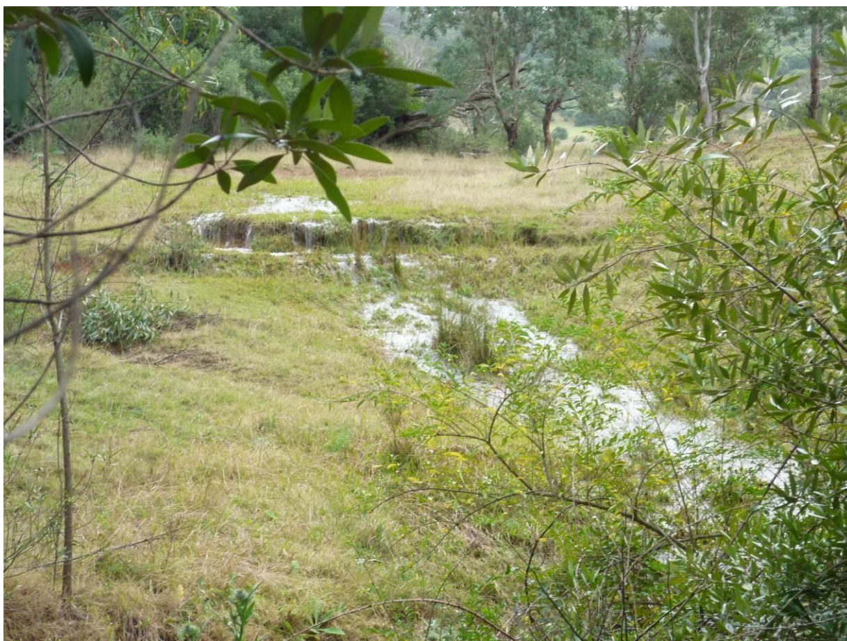
Photo 11 – Spillway for Dam 2 - requires stabilisation
